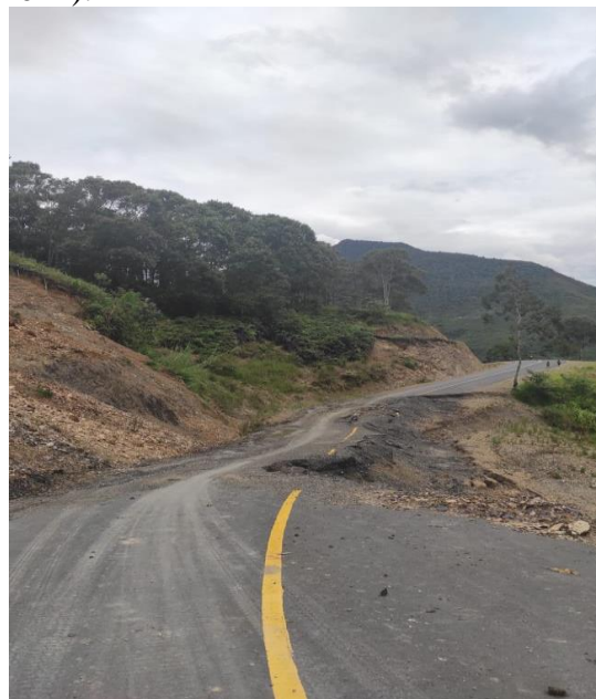
Figure 2. Road Damage: Ruts (Survey 2021)
