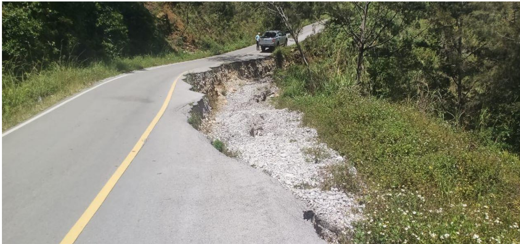
Figure 3. Road Damage: Grade Depressions (Survey 2021)
