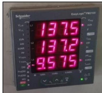
Figure 5 Power Meter Analyser Schneider EasyLogic™ PM2100
