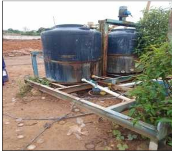
Figure 4. Chemical Organic Coagulant Reservoir
