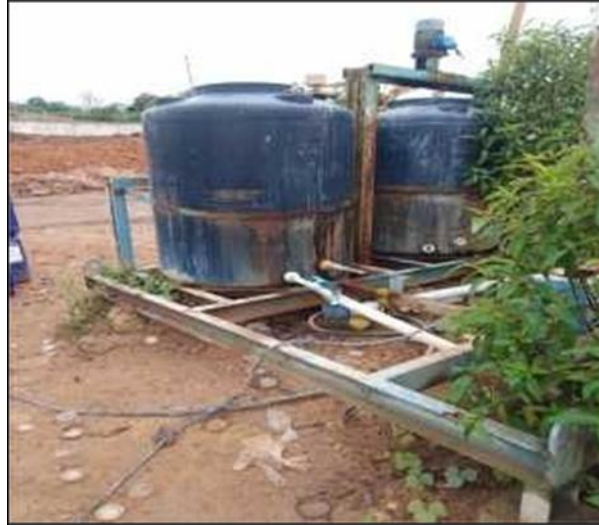
Figure 4. Chemical Organic Coagulant Reservoir
