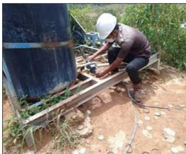
Figure 10. Chemical Organic Coagulant Discharge Measurement
