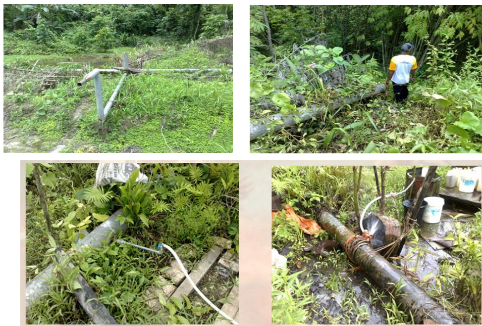
Figure 3. Illicit tapping on a transmission pipeline
