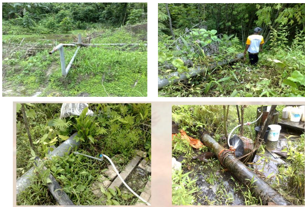
Figure 3. Illicit tapping on a transmission pipeline
