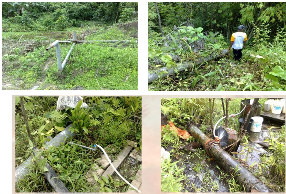
Figure 3. Illicit tapping on a transmission pipeline
