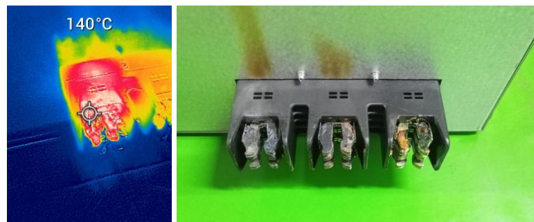
Figure 3 Excess heat causing damage to part of MCC Equipment
