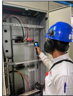
Figure 2 Actual Monitoring Measure Temperature MCC
