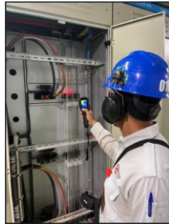
Figure 2 Actual Monitoring Measure Temperature MCC
