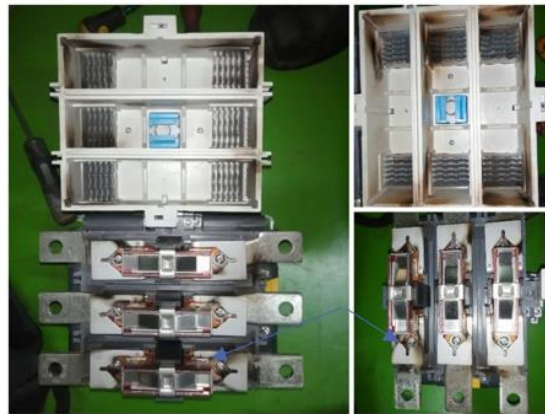
Figure 6 Condition of the arching chamber and the surface of the contactor
